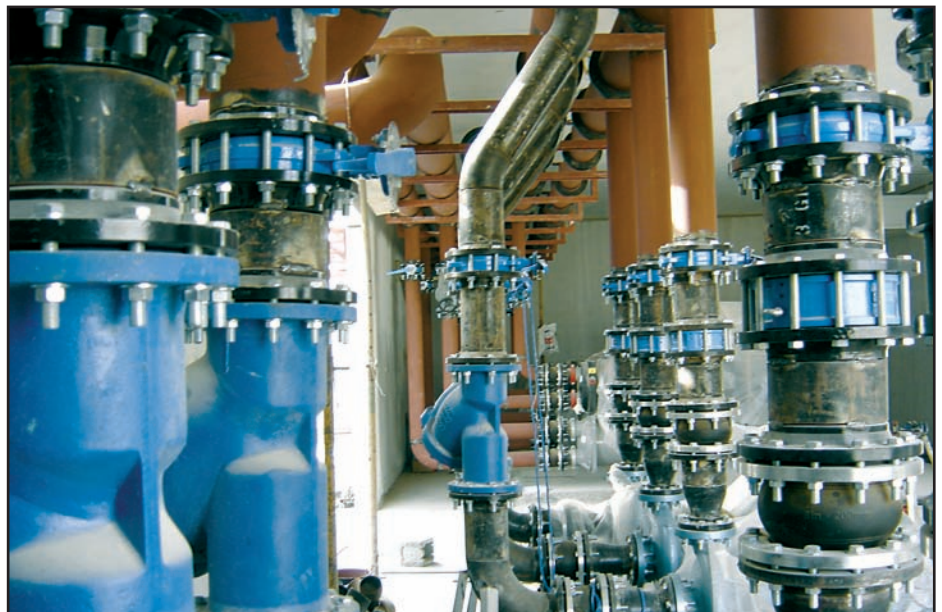
All HVAC equipment, lighting, access control, and facility management software are fully integrated onto a Web-based BAS and situated on a fully converged IP backbone.
