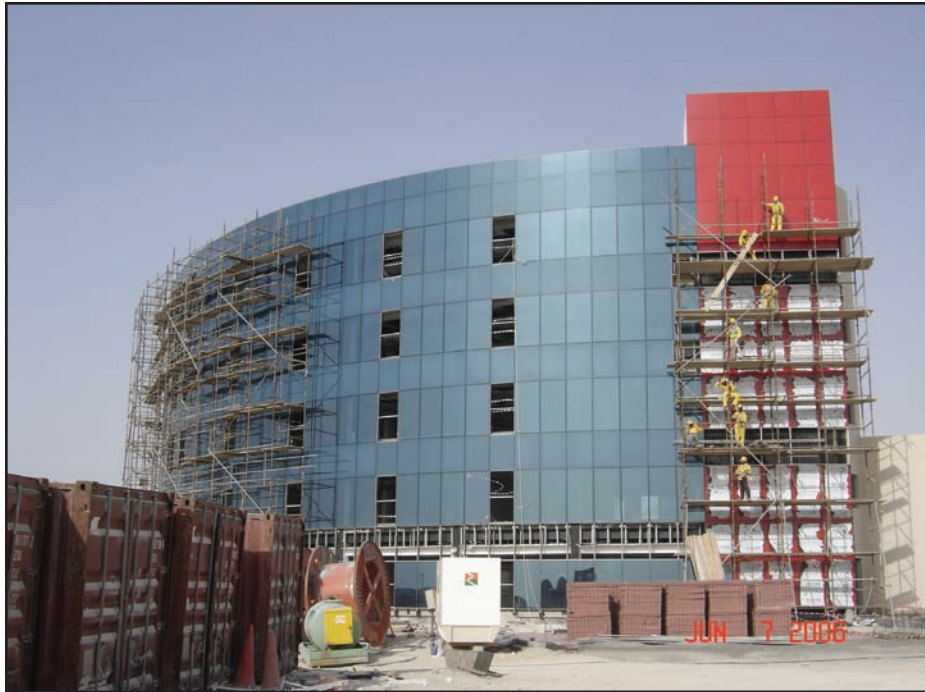
PCS' new facility in Dubai, the first LEED® building in the Middle East, features solar thermal A/C, water-efficient equipment, VSDs and CO 2 monitoring.
